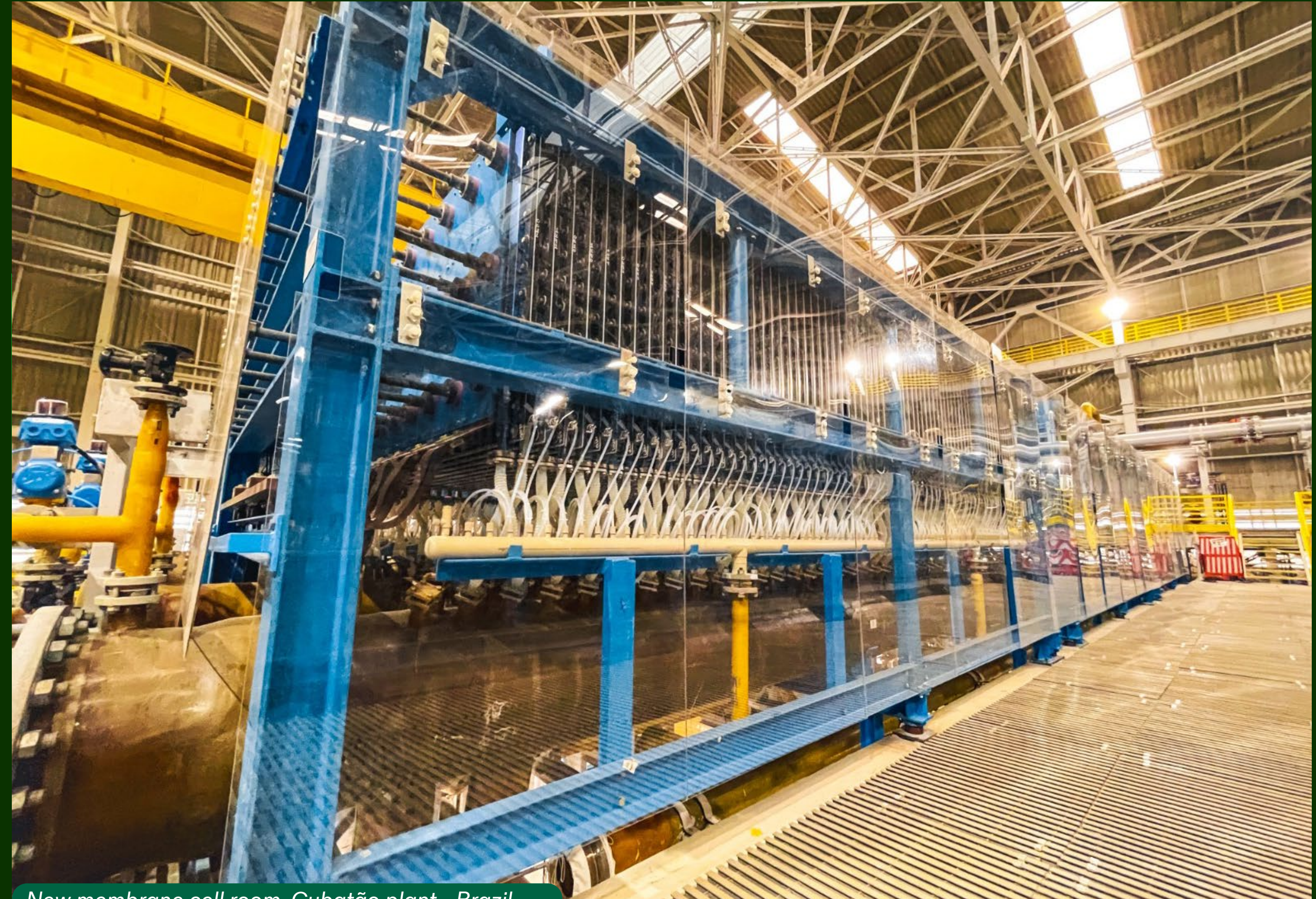
New membrane cell room, Cubatão plant - Brazil
